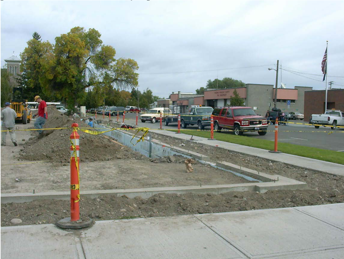
This commercial strip under construction in the heart of downtown is one example of infill development.
